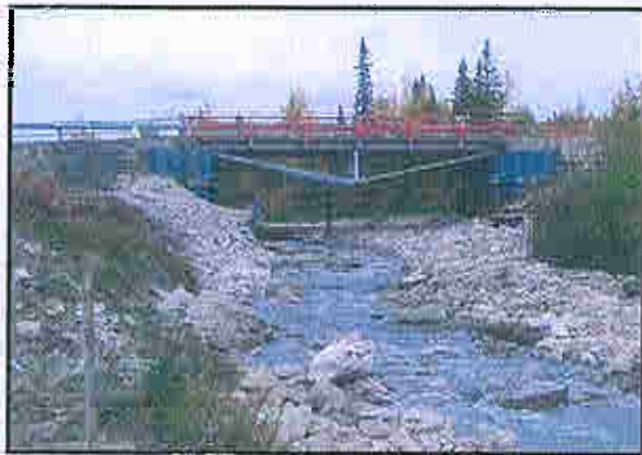
The lower bridge following removal of the weir in 2005 (above). Successful restoration of downstream habitat. Photo courtesy of Imperial Oil Resources Ltd.
